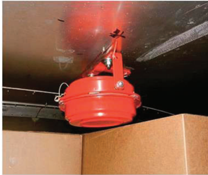
Figure 6.2. In-container fire suppression system
